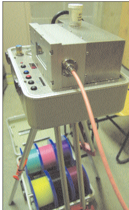
Compressed air is delivered to propel up to 12 optical fibers through each Microduct tube.
